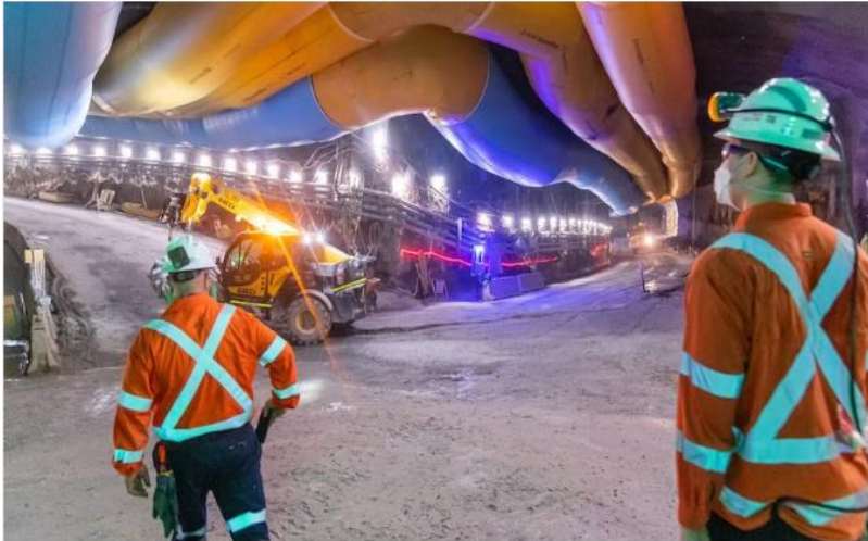
Worker shortages are threatening investment, according to Infrastructure Australia. (Supplied: Transport for NSW)
